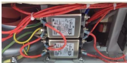
Two EMC filters fitted, Heater & Microwave*
