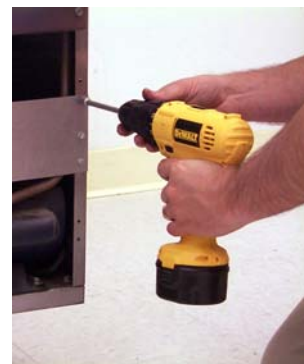
Removing gas manifold shield.
