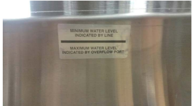
Water Level Decal Located on Front of Tank
