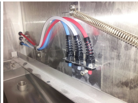
Chemical inlet tubes
