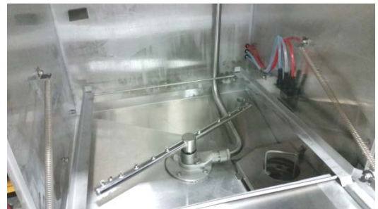
Wash cabinet and wash arm
