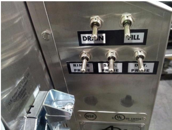
Showing controls on lower access door
