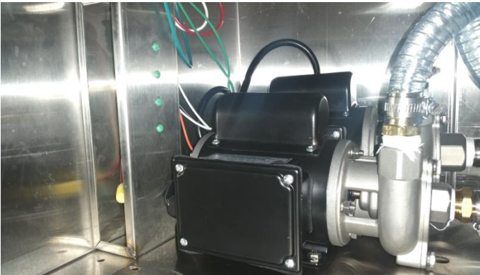
Wash pump is placed behind the rinse pump shown here
