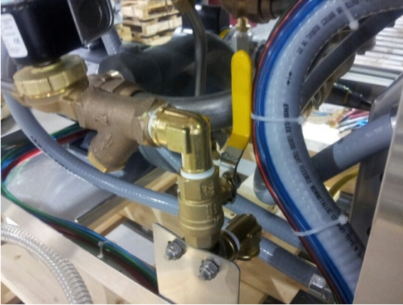
Showing \frac{1}{2} " female pipe inlet, ball valve, y-line filter, H2O solenoid
