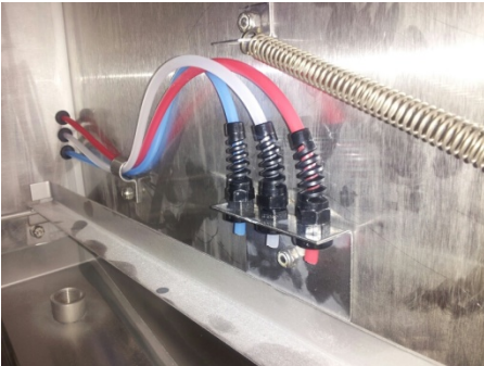
Showing chemical lines above sump
