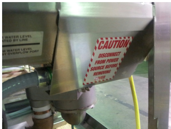
Heater terminal box in right front side of the pan
