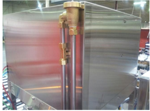
ASSE approved vacuum breaker (backflow preventer)
