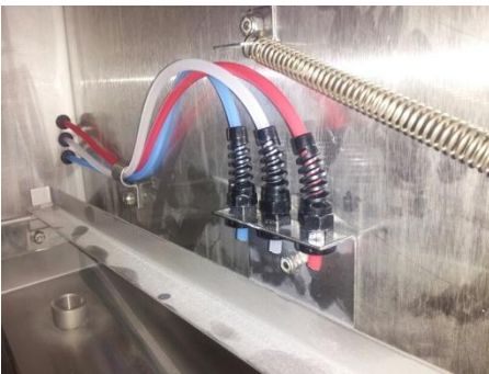
Showing chemical lines above sump
