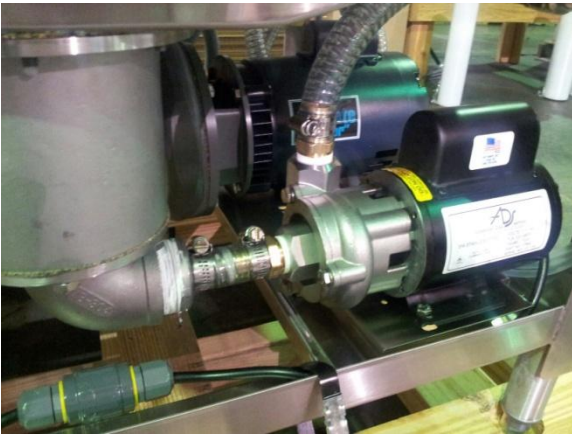
Showing stainless drain pump w/3/4" discharge tube
