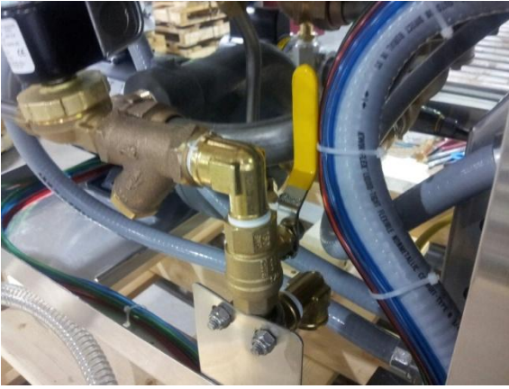
Showing 1/2" female pipe inlet, ball valve, y-line filter, H2O solenoid
