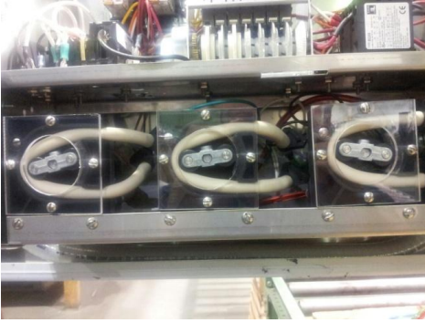
Showing deter, rinse, sanitizer internal chemical pumps
