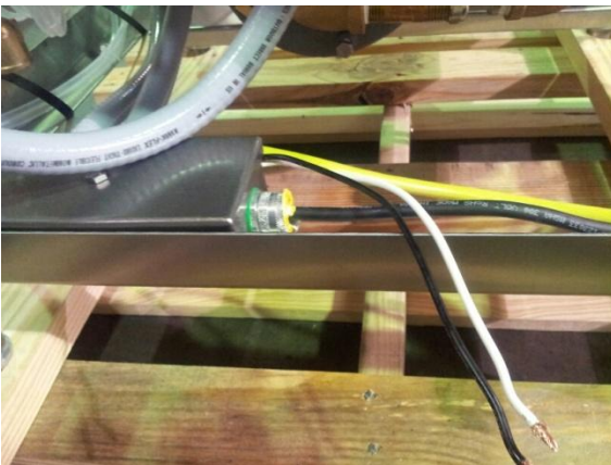
Power junction box for incoming 120v power
