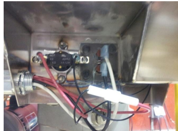
Heater box less cover, thermostat, element, float wires
