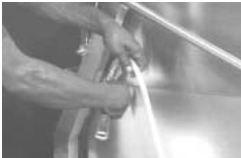
Use pipe dope, then connect and tighten the spray hose to the front of the faucet
