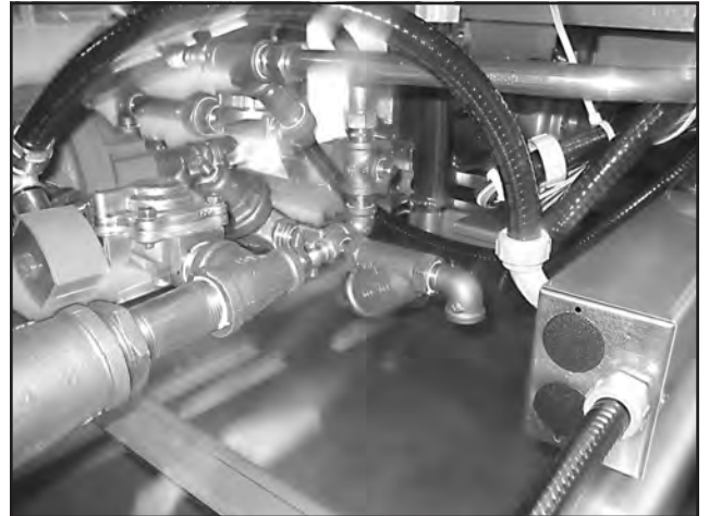
Hot water connection
