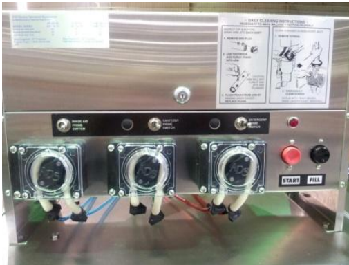
Showing deter, rinse, sanitizer external pumps
