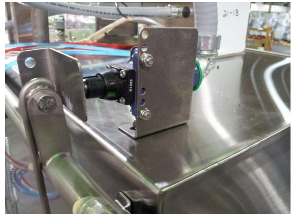
5-CD Door cut-off switch and lever arm
