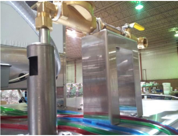
Showing hot water inlet, solenoid, and air gap
