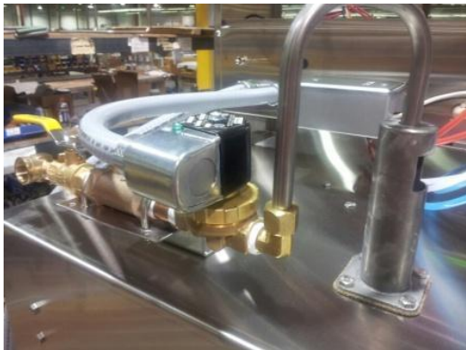
Showing ½” female pipe inlet, ball valve, y-line filter, water solenoid, ASSE approved air gap (backflow preventer)
