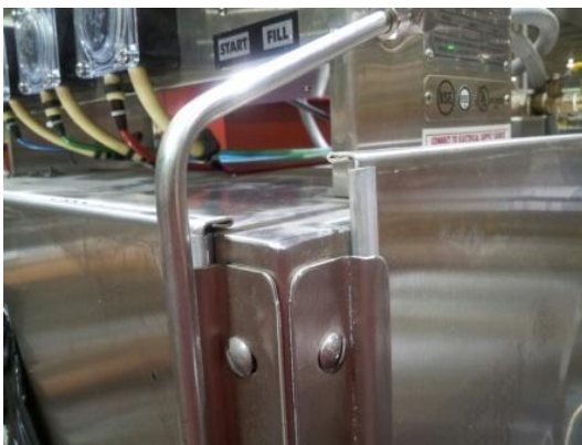
Showing misaligned arms
