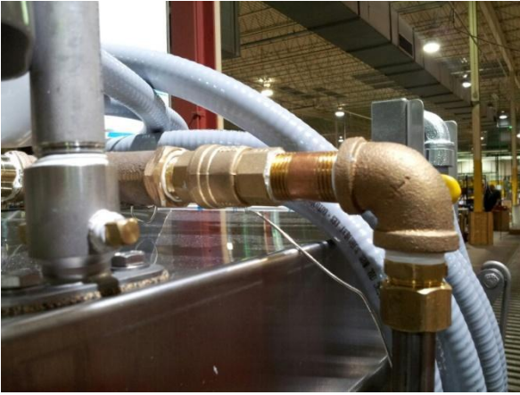
HT hot water inlet ball valve, connected to booster line
