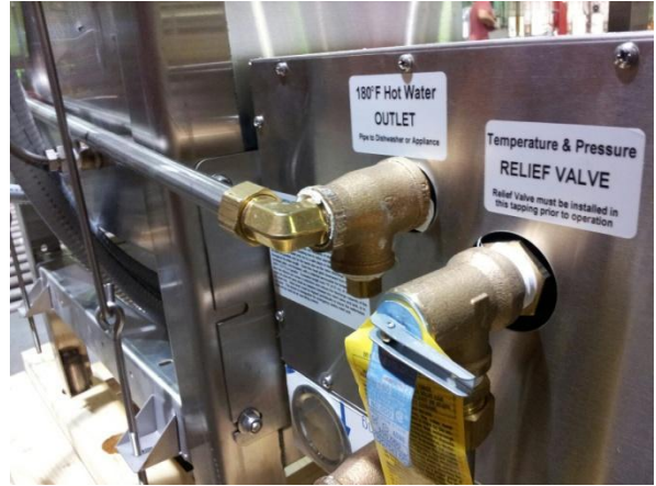
Booster hot outlet line going up to HT-25 inlet manifold
