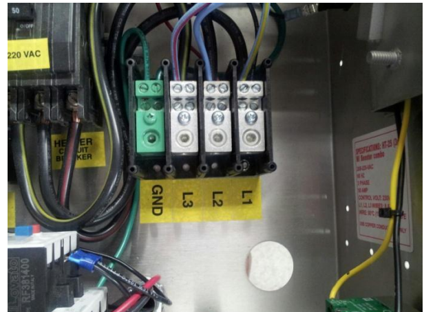
Main distribution block for incoming wire & 1” conduit hole
