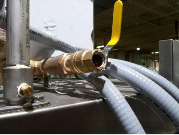
Showing final rinse mixing chamber, hot-water inlet to HT-25
