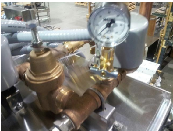
Showing pressure reducing valve for final rinse & gauge*
