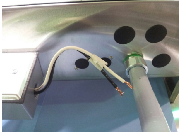
Showing power connection box for 120v wiring
