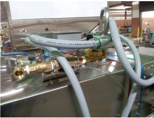
Showing 1/2" female pipe inlet, ball valve, y-line filter, water solenoid,
