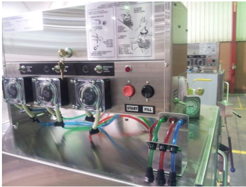
Showing deter, rinse, sanitizer external pumps
