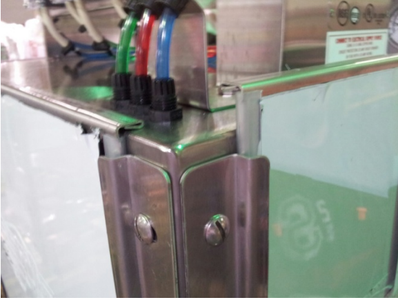
Showing ❌ misaligned arm, same is true for inline
