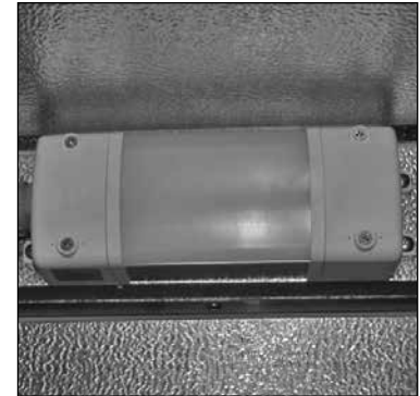
LED light fixture
