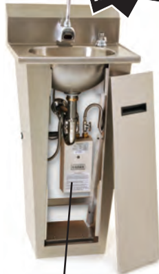
hot water heater
