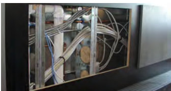
removable front panels expose the chase for repairs and modifications.
